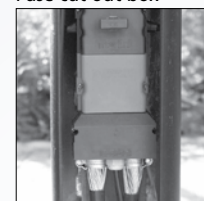
Fuse cut out box
