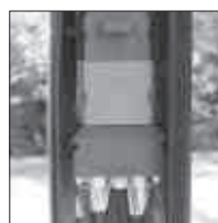
Fuse cut out box
