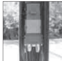
Fuse cut out box
